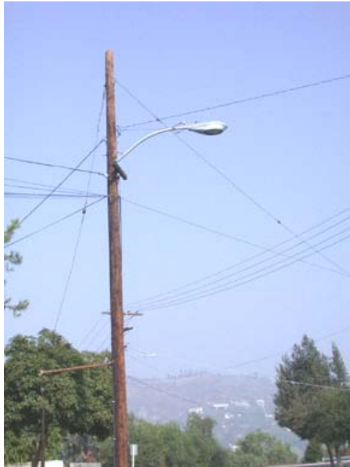
In-Fill Street Lighting
